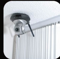
監控設備 附設遙控及錄影 CCTV (with Remote and Recording)
